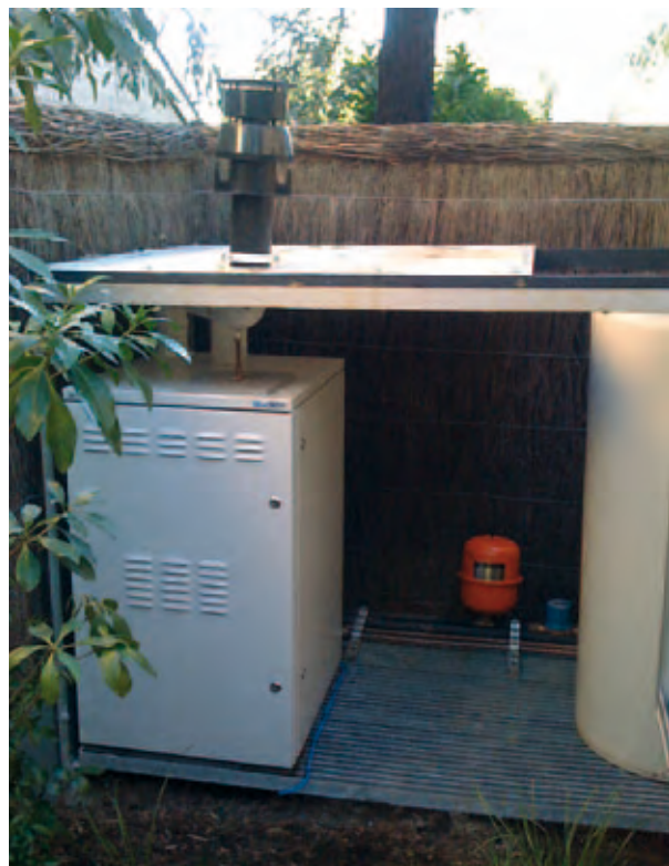
BlueGen installation at Energy Australia's Smart Home in Newington, Sydney.
