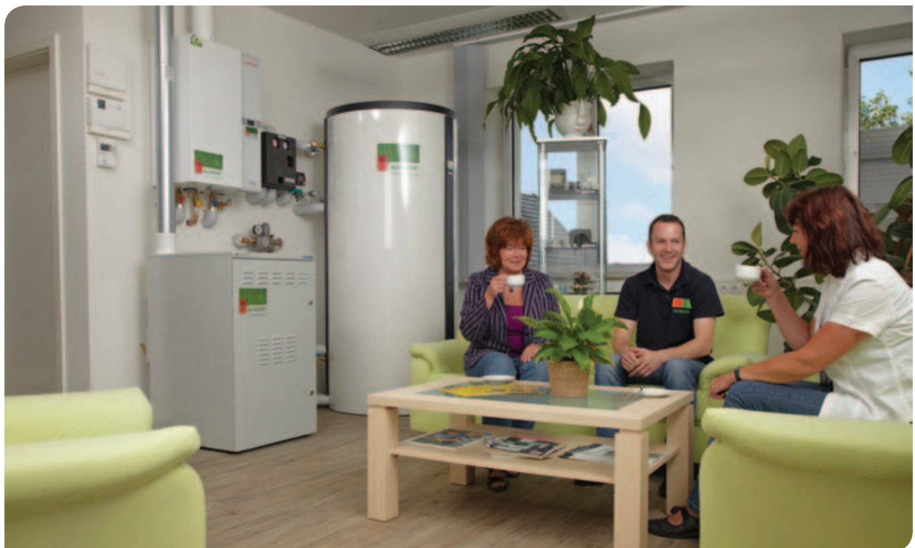
▲ Installed in the German offices of Alliander Netz AG, BlueGen integrates with the building's hot water tank and heating system
